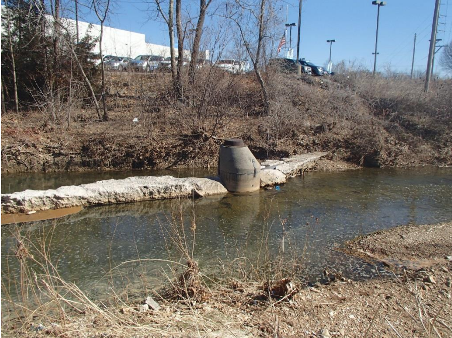
Exhibit 1 – Photographs of the Exposed Manhole and Sanitary Sewer Piping
